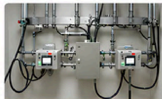
Gas Manifold System
