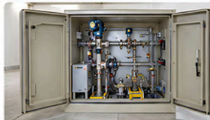
Process Instrumentation Enclosure
